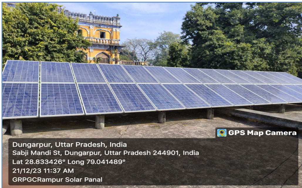
Picture 7: Rooftops Solar Power system installed in the College premises
